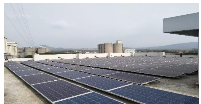
Figure 9. A rooftop Solar Power Plant
