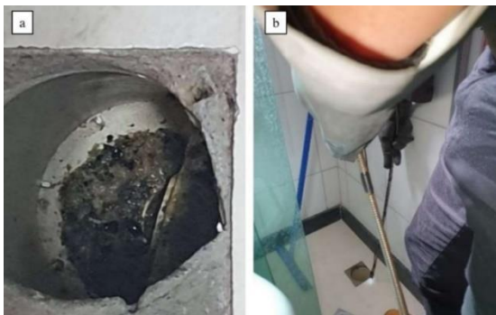
Figure 3. a) Siphoned drain with presence of waste water, b) Attempt to inspect the siphoned box drain
