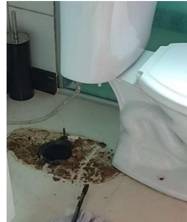
Figure 4. Removal of the toilet bowl and evidence of effluent backflow
