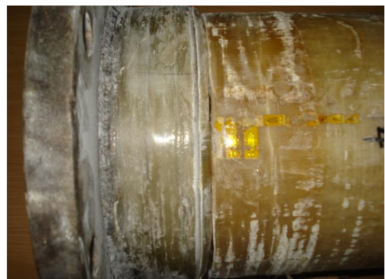
Figure 4 Shows the area of the flange forms the brink of collapse
