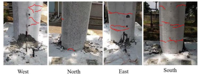
Figure 12. Crack pattern of SPPC 03 specimen
