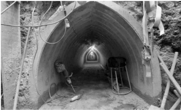
Figure 5. Bullet tunnel(140m in length, 1,6m tall e 1,5m de wide)was intended for rainwater collection. (Estado de Minas, August 2018)
