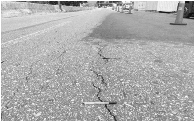
Figure 2. Cracks detail on the crest of the slope. (Image courtesy of Thiago Bomjardim Porto)
